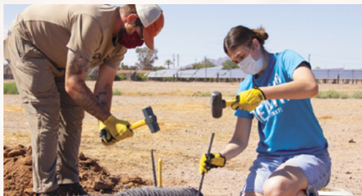
Tyler Obermeit, '21 BS applied biological sciences, and Zahra Husrieh install rebar into each side of a burrow entrance.
